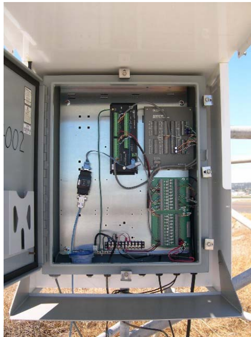
Figure 5. Data logger system housed inside equipment box.
