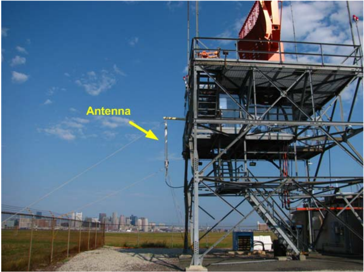
Figure 15. Antenna installation for Logan measurements
